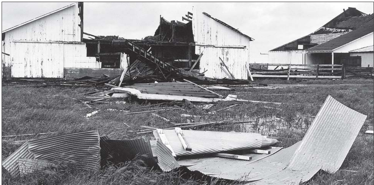
Photo 1-3. High winds estimated at 100 mph have done major damages to these farm buildings.
