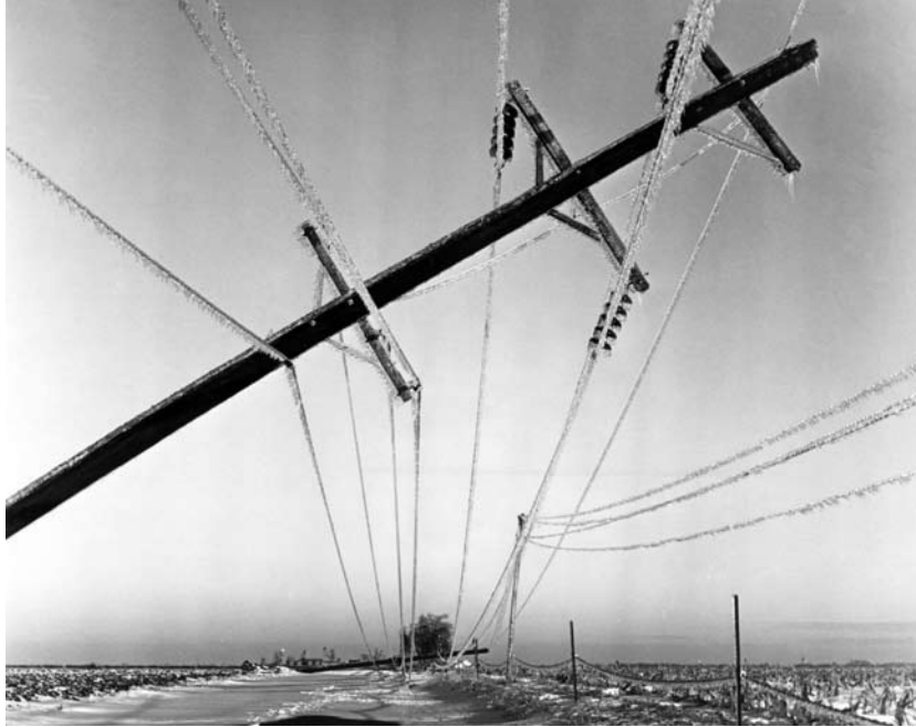
Figure 2-8. The massive ice storm in Illinois and Missouri tore down many power poles, including this one in rural western Illinois on December 2, 2006.
