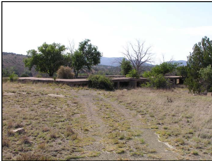
Figure 9. Front foundation of the second hospital at Fort Bayard (view is northeast). First hospital was located to the right and down the knoll. Photograph by author (August 2005).
