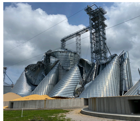
Derecho winds flattened corn crops and collapsed grain bins in Iowa.
