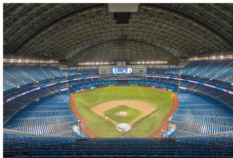
Rogers Centre, Toronto, ON. Roof was damaged in April due to Ice Accumulation.
